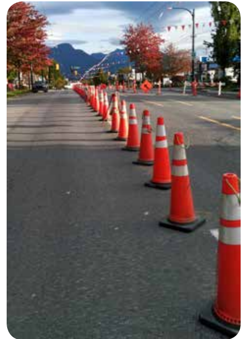
Traffic cones today, new sewer pipes for the next century – and then a surprise!
